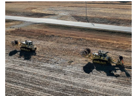
K & H Electric uses tandem dozers to rip and drop the power lines.
