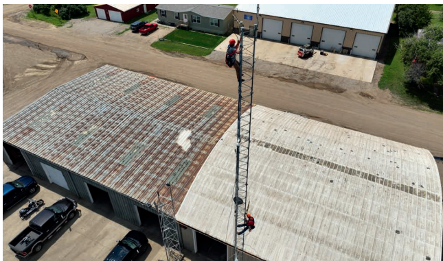
Eric and Andy of Rushmore Communications removing antennae and cables from the tower.
